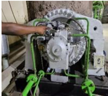
Figure 15. NFC based equipment local visits/inspections.
